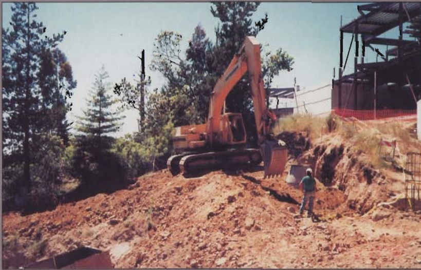
Steep grades required excavators to construct job site access areas. (Photo: Perretti & Park Pictures)
