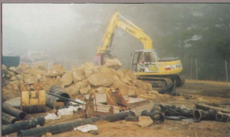
Fog and boulder removal were another construction challenge. (Photo: Perretti & Park Pictures)
